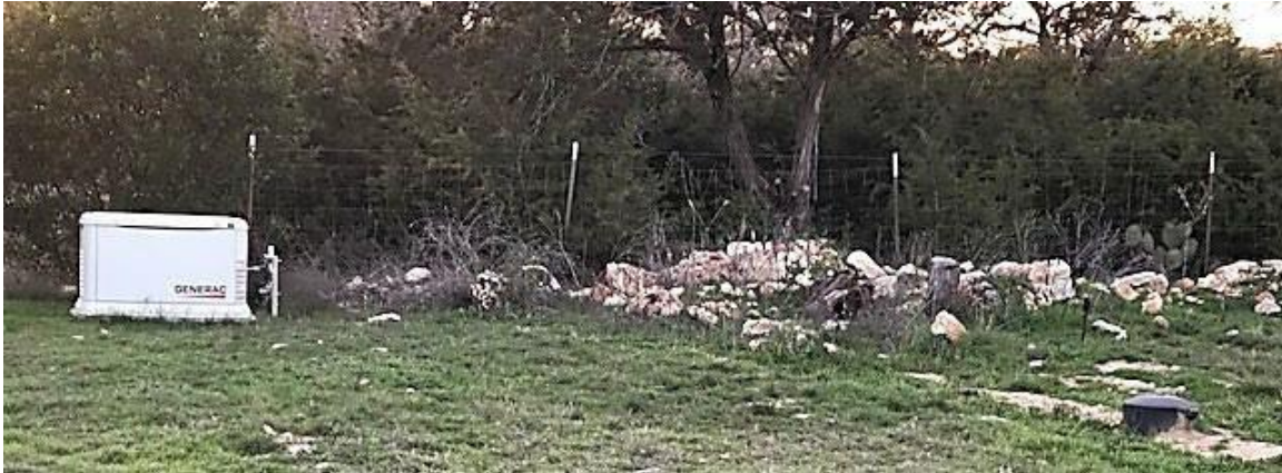
Figure 23. Generac 22 kWh whole-house generator and propane tank
