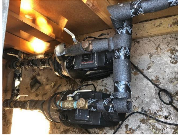
Figure 11. Parallel on-demand pumps
