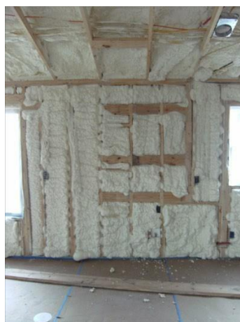
Figure 5. Open-cell spray-foam insulation
