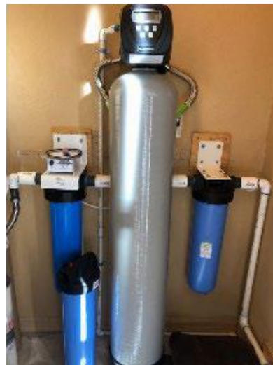
Figure 12. From right to left: sediment filter, charcoal regeneration, ultraviolet filter (spare tank in front)
