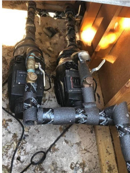
Figure 11. Parallel on-demand pumps
