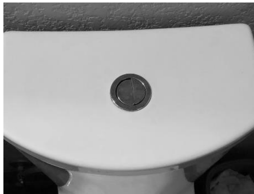
Figure 15. Low flow (dual flush) toilet, installed
