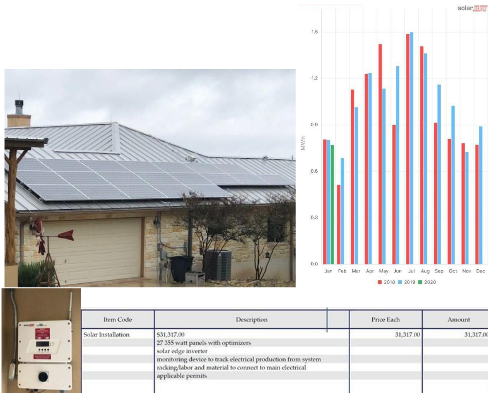
Figure 19. 10 kWh SolarEdge system (top left) with inverter (bottom left), power production (upper right), and acquisition costs (lower right)
