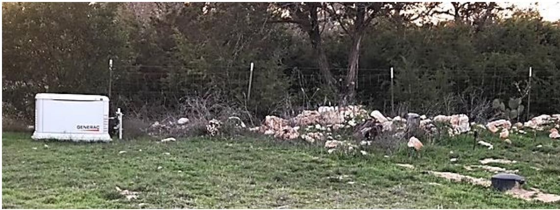
Figure 18. Generac 22 kWh whole-house generator and propane tank
