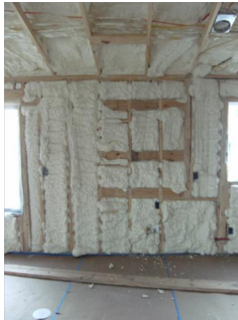
Figure 5. Open-cell spray-foam insulation
