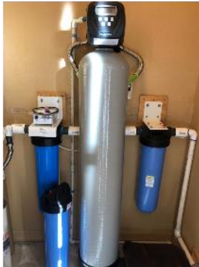
Figure 12. From right to left: sediment filter, charcoal regeneration, ultraviolet filter (spare tank in front)
